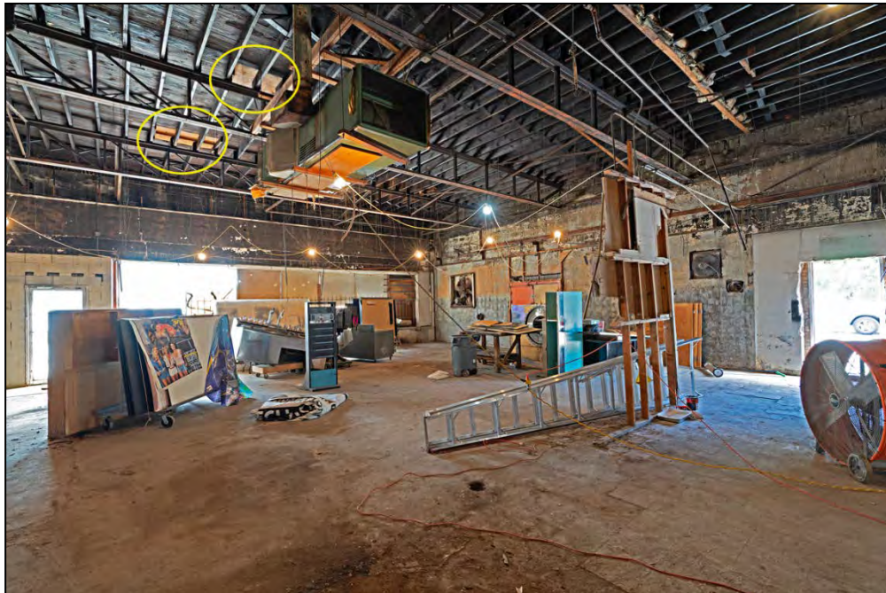
Figure 11: The yellow circles highlight examples of roof damage at the west central (top) and east central (bottom) portions of the building, 2022.
