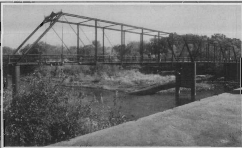
The Caplinger Mill Bridge (ca 1885) in Cedar County is an example of a Pratt, through-truss bridge, the most common truss type in the nation. This particular bridge is unusual because it has had few alterations and still retains its decorative portal bracing and strut and its distinctive bridge plate. It is also part of a once-common Ozark development pattern consisting of bridge, mill, and store forming a hamlet. Progress has caused most of these hamlets to grow into today's town or to vanish.
