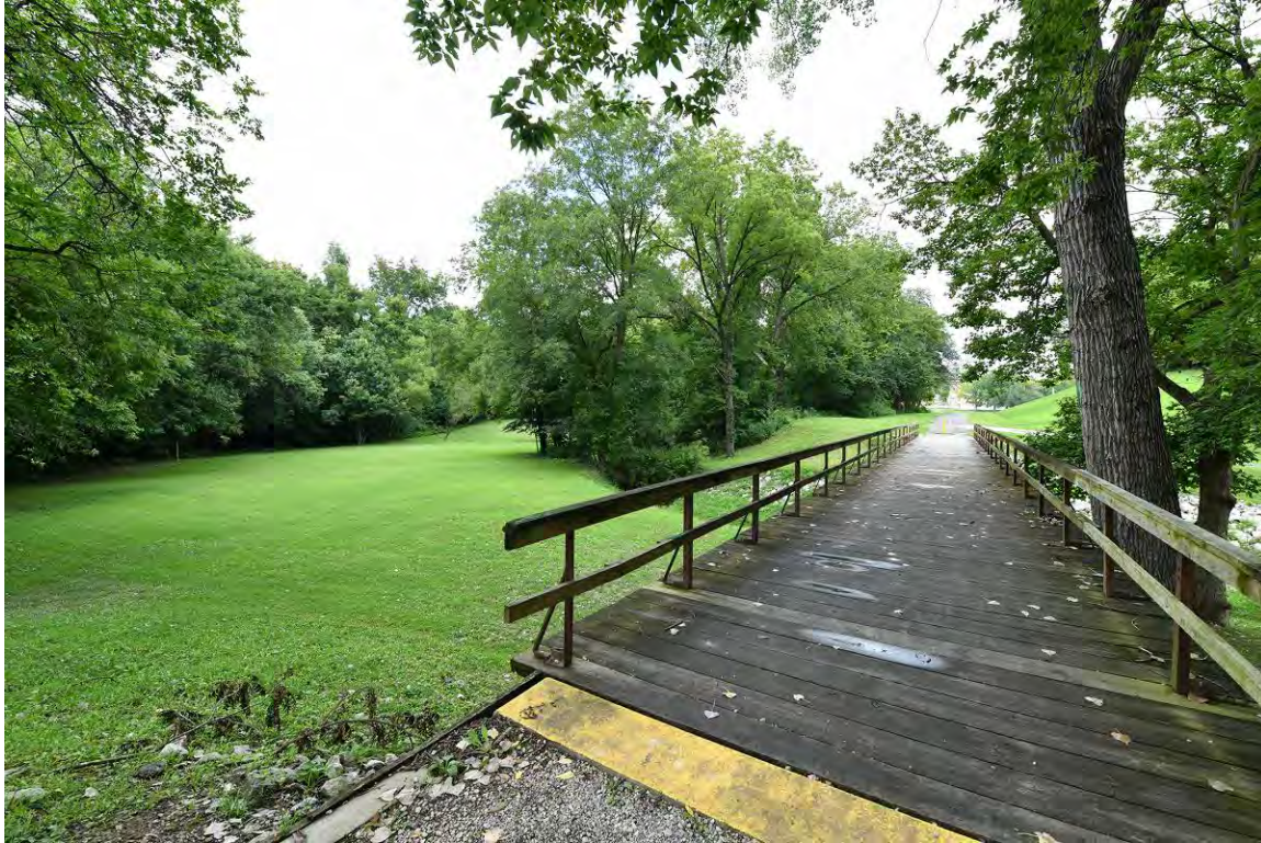
Figure 28: Rupe Branch Bridge ( Resource 28 ), showing wood deck and railing, looking east (Brad Finch, f-Stop Photography, 2023).
