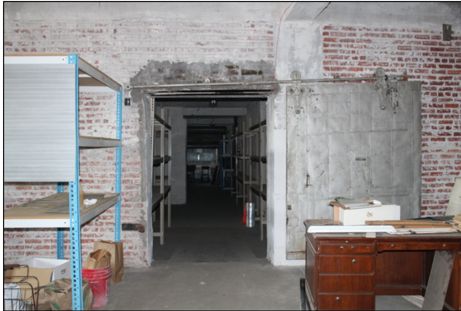
Figure 31: Example of fire door egress at the third story, 2022. Source: Kelsey Lutz, photographer.
