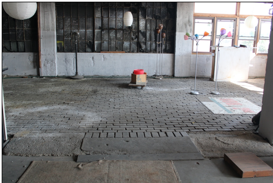
Figure 33: Third floor, view facing north, area with brick flooring and concrete ramp, 2022. Source: Kelsey Lutz, photographer.
