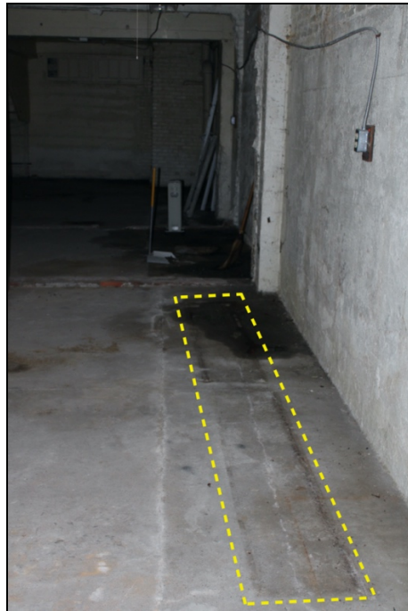
Figure 35: (Top, Left) Original floor drain for parts washing system (covered with wood for safety). (Top Right) Remnants of the parts washing system tie ins with soil pipe. (Bottom) The yellow dashed line indicates the location of the infilled floor basins.
