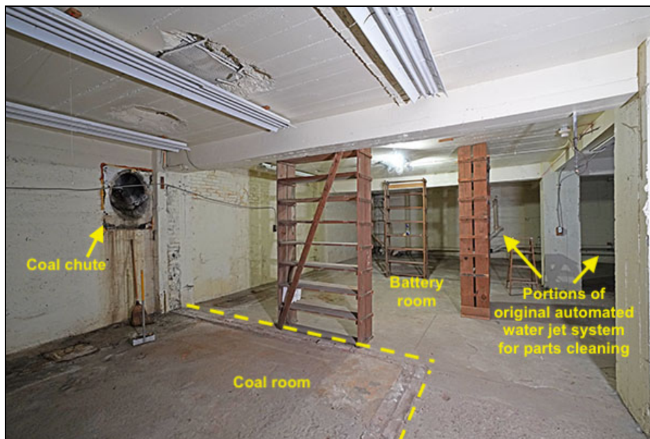
Figure 34: Labeled view of a portion of the basement level, view facing northeast, 2022. Source: Richard Welnowski, photographer; photo labeling Kelsey Lutz.
