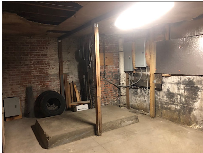
Figure 30: (Top, Left) Yellow arrows point to the original partitioning of the Dynamo Room at the northwest corner of the first floor. (Top, Right): remnants of the dynamo's connection to overhead electrical (alternating current) lines on the north façade. (Bottom) Interior of Dynamo Room with concrete platform. All photos taken 2022.
