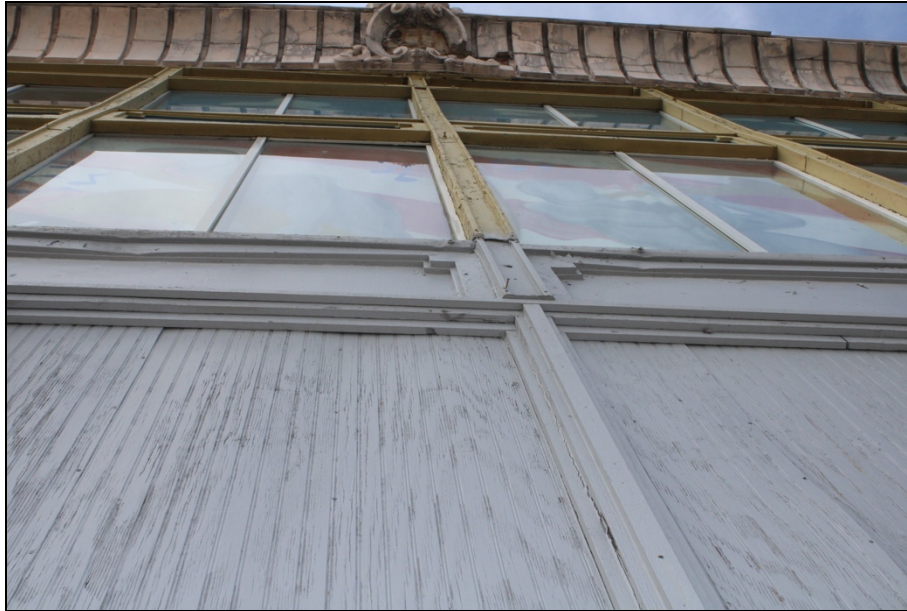
Figure 25: Exterior, east façade, detail of curtain wall system, 2022. Source: Kelsey Lutz, photographer.
