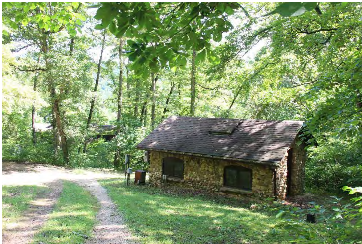
Photo 18. Pump House. Camera facing north. The maintenance road can be seen in the foreground. (Deb Sheals, 2019.)
