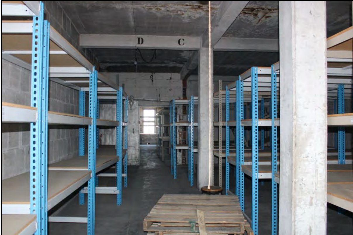
Figure 29: Interior, sixth floor, typical view of larger storage area with rolling fire door. Source: Kelsey Lutz, photographer.
