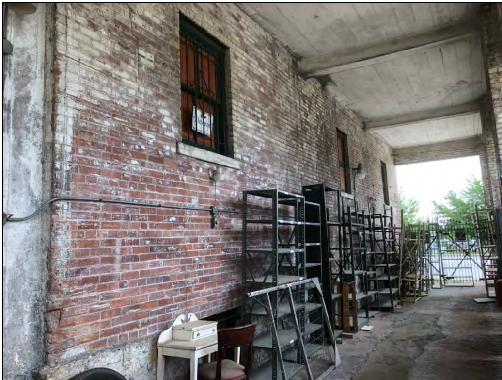
Figure 26: Original dock area, now a through bay at the south elevation; view facing northeast, 2022.
