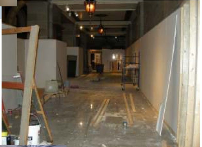
Dry wall is up and getting ready for its fresh coat of paint
